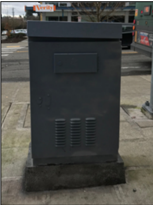
STANDARD UTILITY BOX ON NW 57TH ST & 24TH AVE NW
