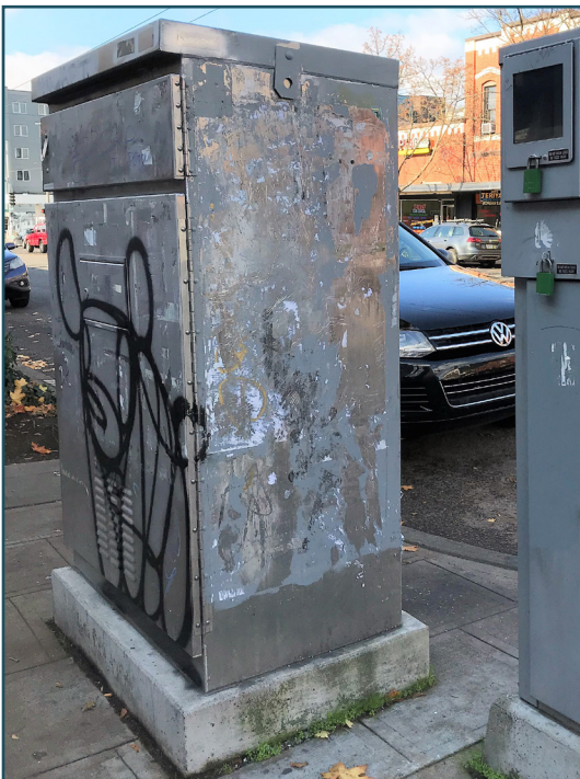
UTILITY BOX ON MARKET ST & BALLARD AVE
